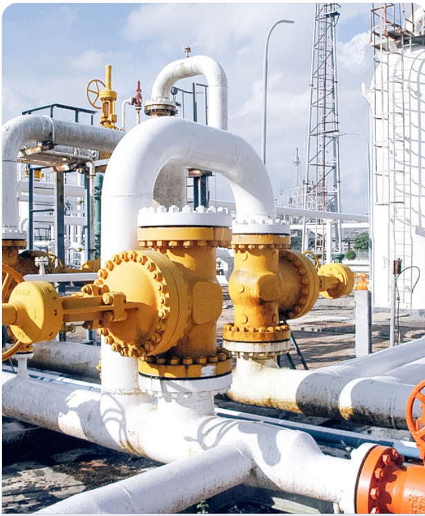
A gas distribution center.
