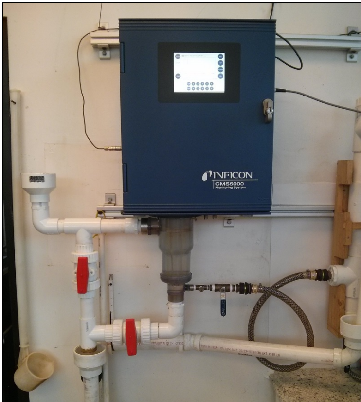
Figure 3: CMS5000 installed at ORSANCO site in Midland, Pennsylvania, USA
