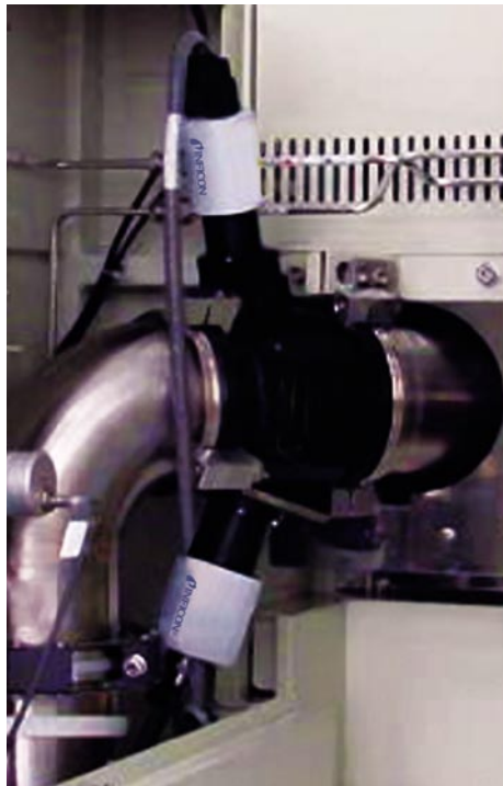
Figure 1 - Stiletto installed in the exhaust of a vertical poly furnace.
